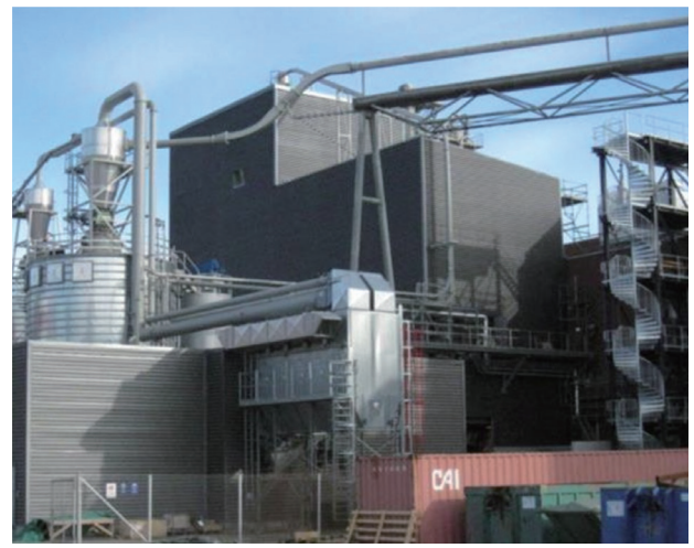
図4 Stora Enso社の酸素-蒸気式流動床ガス化炉 Oxy-steam Fluidized Bed Gasifier of Stora Enso (Finland)
