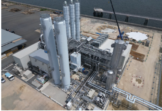
LAES(Liquid Air Energy Storage)
