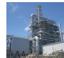
CFB Boilers (Circulating Fluidized Bed Boilers)
