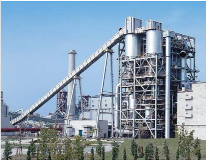
IPP (Independent Power Producer) Coal fired Power Station with CFB
