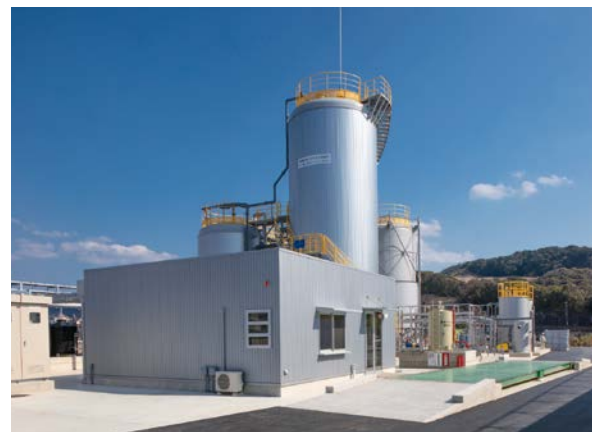
Wastewater treatment system (Anaerobic effluent treatment system)
