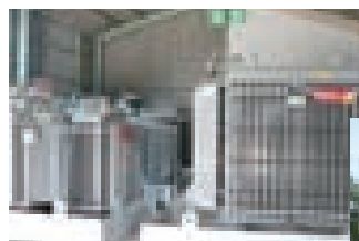
Storing transformers containing minute amount of PCB
