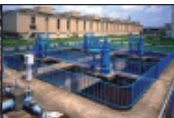
Waste water treatment
