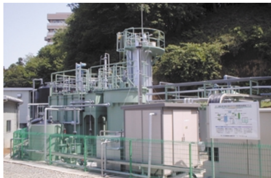
Raw Sewage Treatment System
