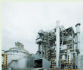
Summit Myojyo Power / Itoigawa plant Steam-generation capacity: 196t/h
