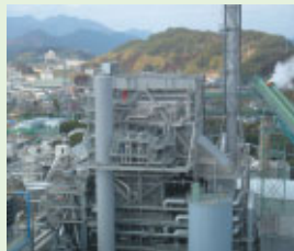
Oji Paper Co., Ltd. / Nichinan plant Steam-generation capacity: 130t/h
