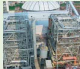
Dragon Special Resin Co., Ltd., China Steam-generation capacity: 3x220 t/h
